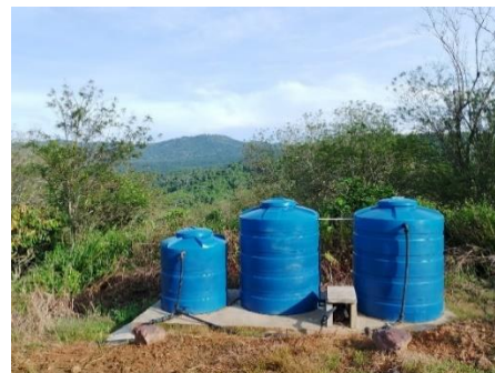
Figure 3: Tanks and water pump platform
